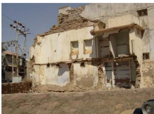
Fig. 3.22 Earthquake damage in Bhuj as seen in Feb. 2005. Photo: N. SLIWA, Feb. 2005
